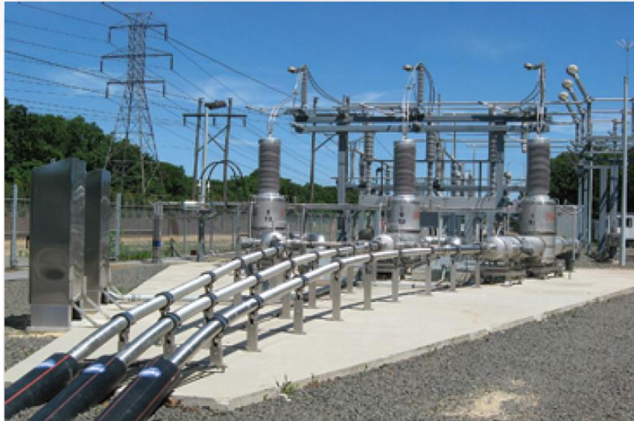
138kV HTS cable system installed in Long Island, NY
