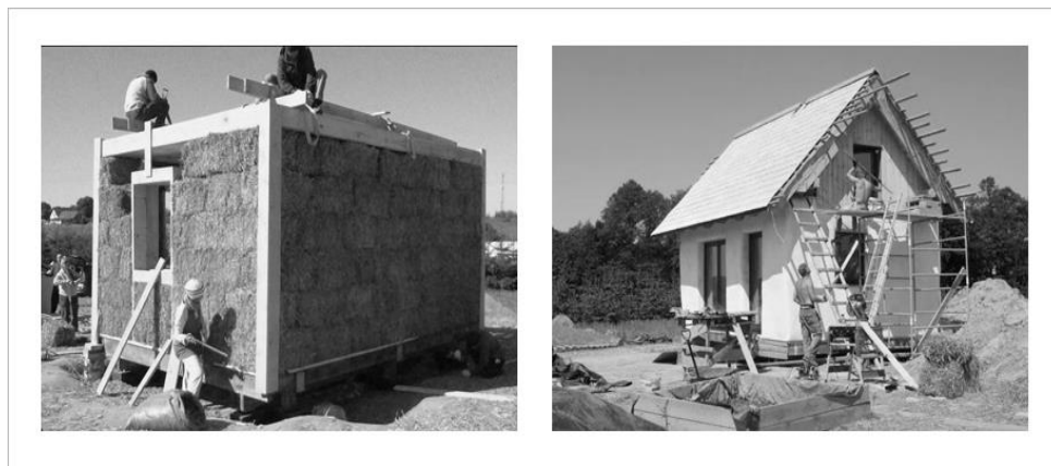
Figure 10. Prototype of open-source house 'Nano-habitat' during a) wall construction, b) plastering. Photo courtesy of Paweł Sroczyński 40
